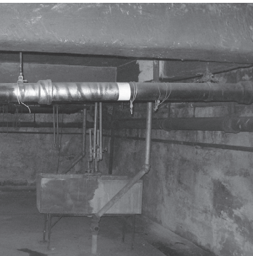
An uninsulated basement heating pipe
